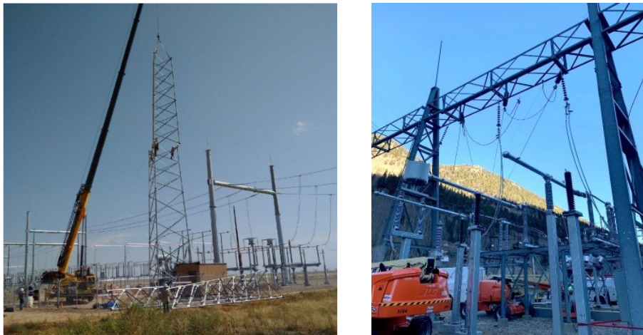
Figure 4. Location of AC induction related accidents: crew erecting a transmission lattice tower near a live 345 kV substation in NM, USA (left), crew replacing a 115 kV circuit breaker on a de-energized line that runs parallel with a 230 kV line CO, USA (right)
