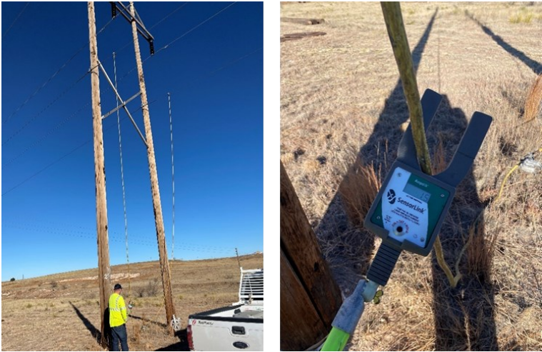
Figure 8. Measurement of AC induced current (1.5 A) with a live tool and a fork type ammeter on the TPG
