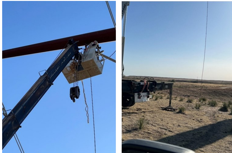
Figure 9. Field trial 2: use of conductive clothing for repairing OPGW over a double circuit 345 kV line with single pole, weathered steel with one circuit deenergized (left); wildfire caused due to flashover of insulating aerial crane outrigger (right)
