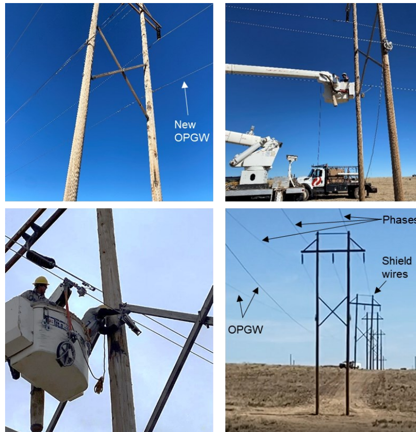
Figure 7. Field trial for use of conductive clothing for installing OPGW under an energized 115 kV line with wood H-frame
