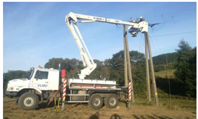
Fig. 1. The location of the accident with the pole and the bucket truck.
